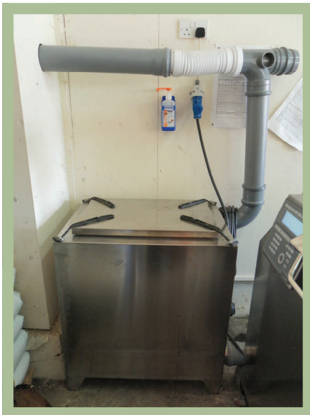
The bio filter unit with outlet pipe
